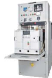
Medium Voltage Panels
