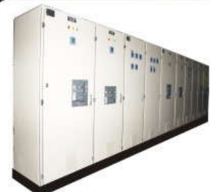
Low Tension Panels
